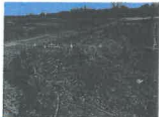
19) Wave action caused approximately six inches of erosion to the top two feet of the landside levee slope. Mow and scarify the damaged slope and place topsoil to return to a 1V on 3H slope. Install erosion control blanket and seed the repaired area.
