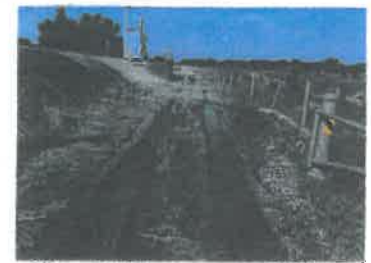
24) Approximately 4 inch ruts in the BNSF berm maintenance road for a 625 foot length. Replace the levee aggregate surfacing on the 15 foot wide maintenance road to elevation 1067.25 feet NGVD29.
