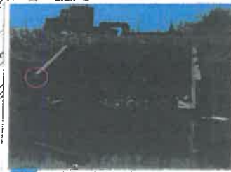
21) A one foot wide, two foot long, and six inch deep spill in the south, riverside wingwall of the box culvert. See the structural drawings for final repair.
