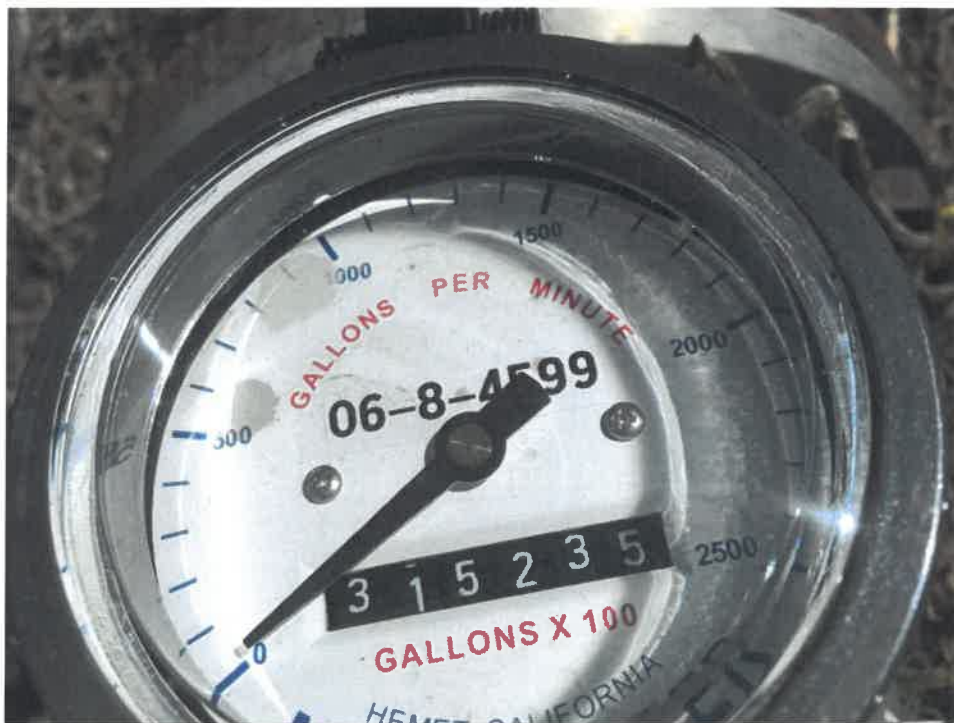
Fig. 11: Meter 06-8-4599 showing meter reading of 315235 gx100 (9/6/2019)
