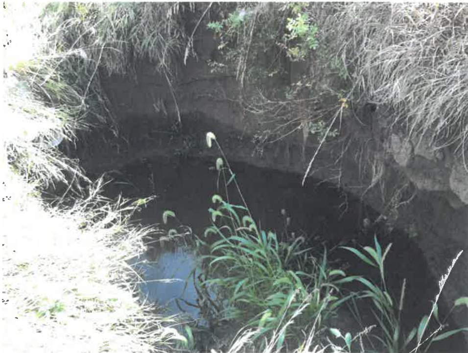
Figure 7: Looking down at puddle of water below tile outlets. (9/6/2019)
