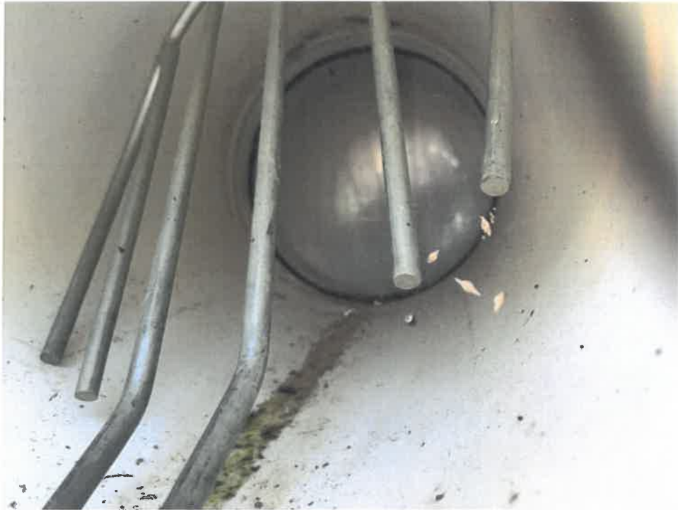
Fig. 6: East outlet pipe with gate closed. (9/6/2019)
