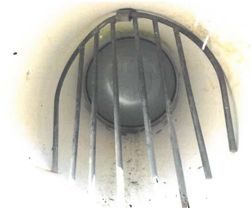
Fig. 5: Middle outlet pipe with gate closed. (9/6/2019)
