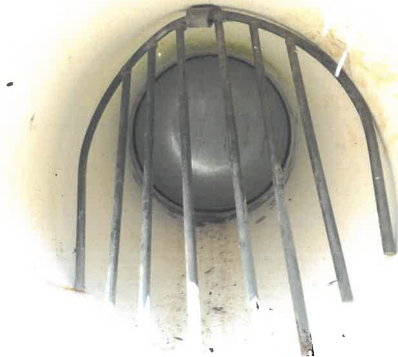
Fig. 5: Middle outlet pipe with gate closed. (9/6/2019)
