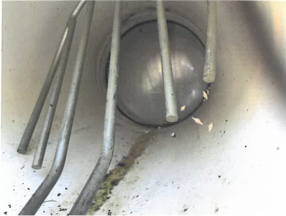
Fig. 6: East outlet pipe with gate closed. (9/6/2019)
