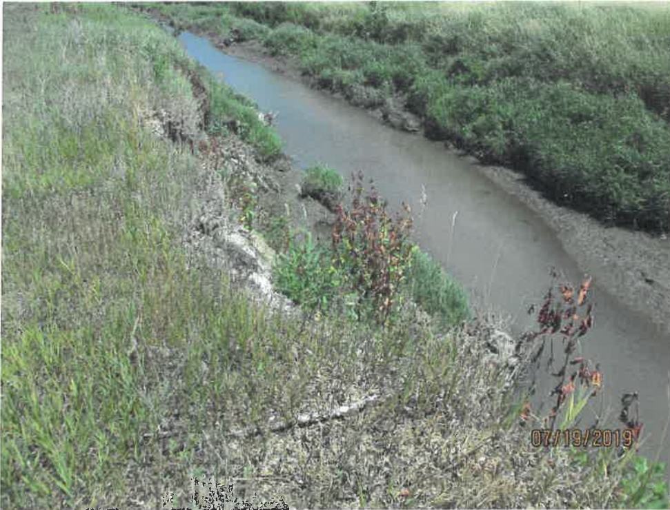
Figure 3: Closer view of failed streambank in Figure 2. Project section is on the left bank in this photo.
