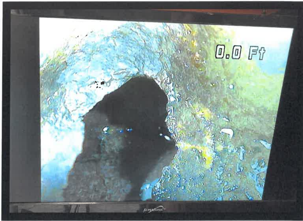
3'-4' into entrance via Antelope Creek floor out outlet. Hole in floor.
