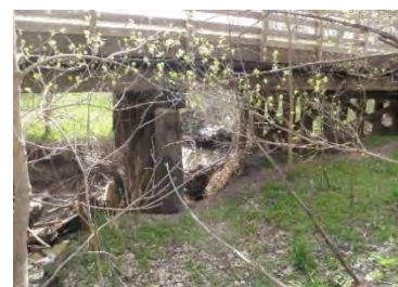
Figure 7-17: Trail Bridge with exposed footings.
