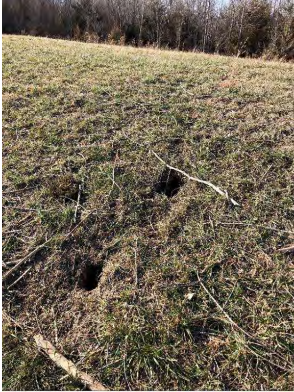
All holes in dam need to be filled
