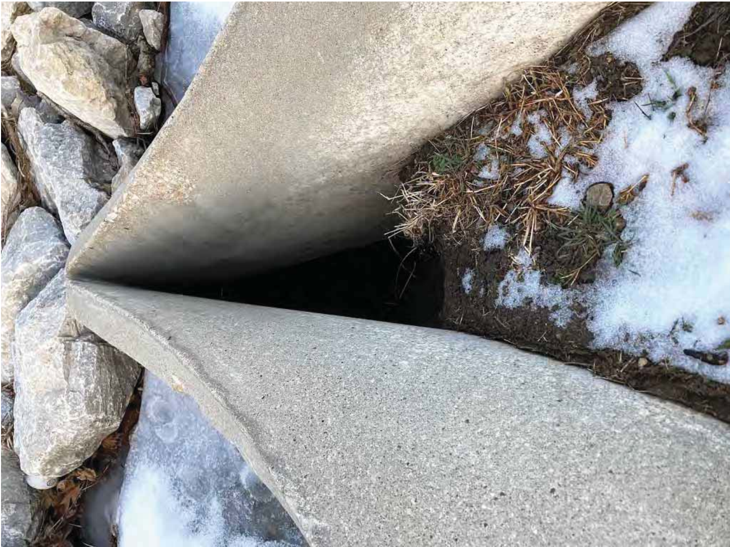
EROSION BETWEEN CULVERTS AT NORTH END
