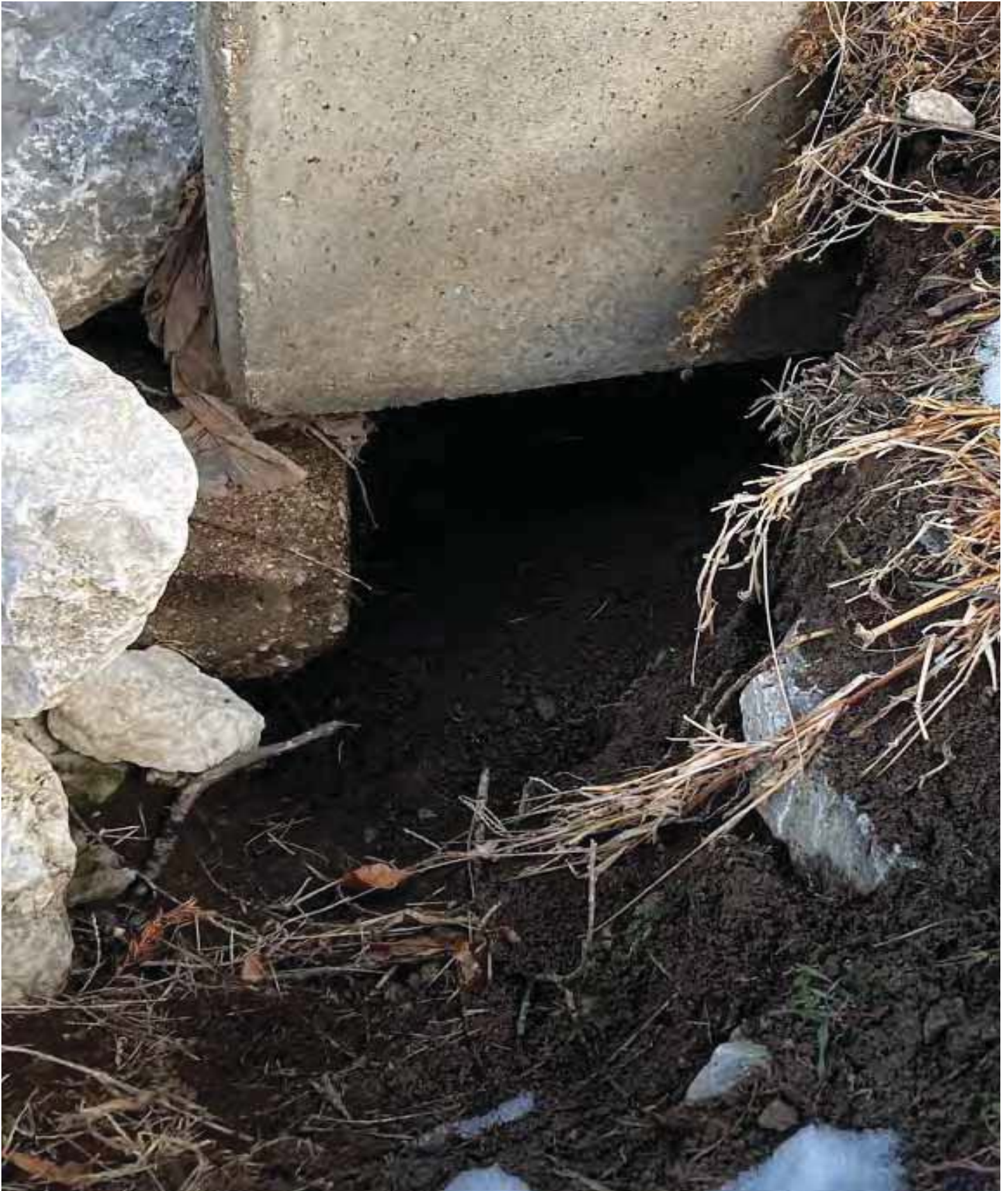
EROSION UNDER LEFT CULVERT AT NORTH END
