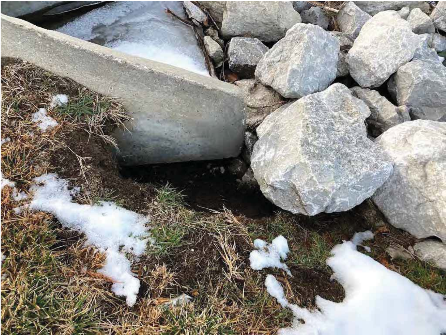
EROSION UNDER RIGHT CULVERT AT NORTH END
