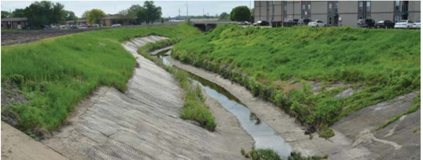
The Deadmans Run Flood Reduction Project will remove nearly 500 homes and businesses from the 100-year floodplain.
