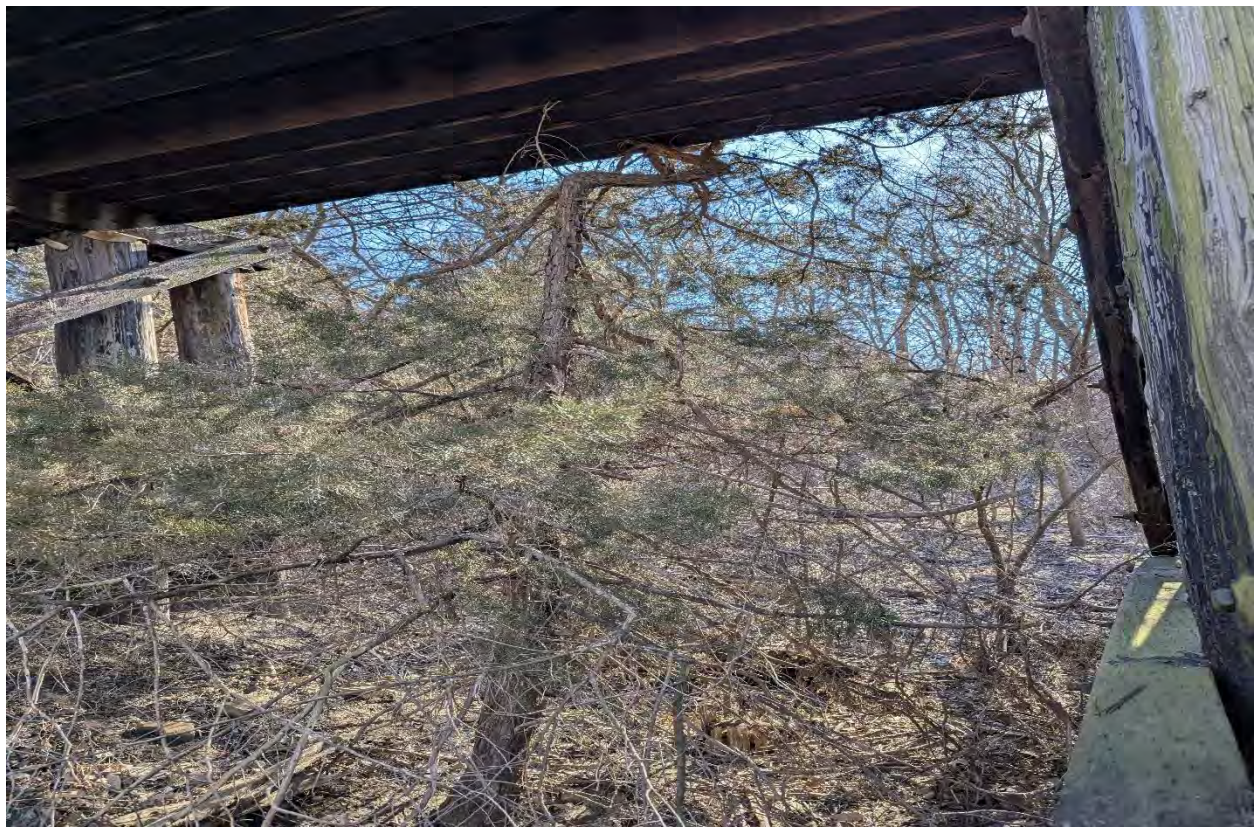
Tree growing into bottom of bridge
