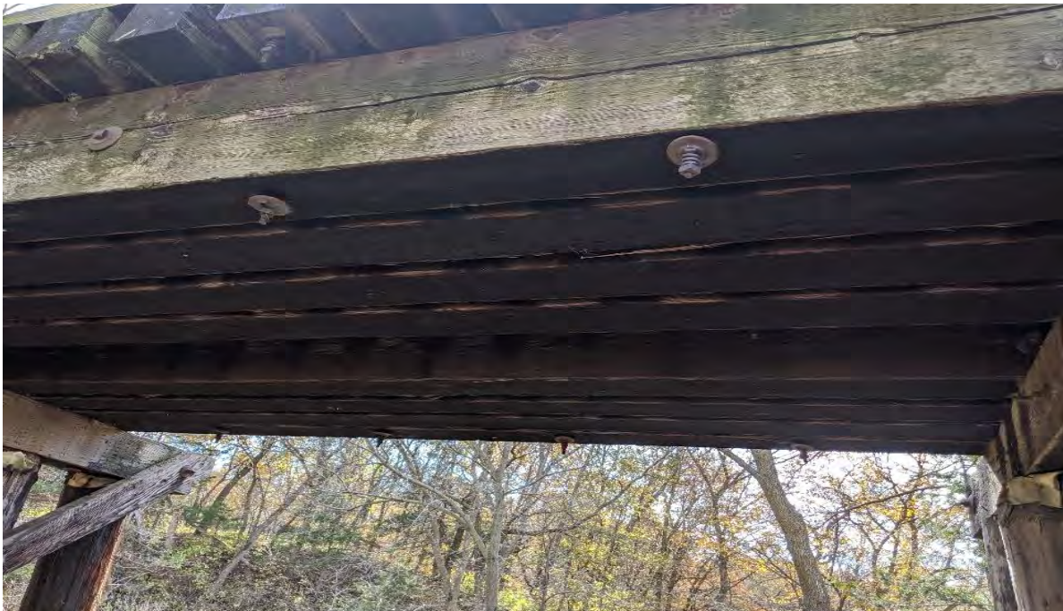
Span, longitudinal crack stringer #1
