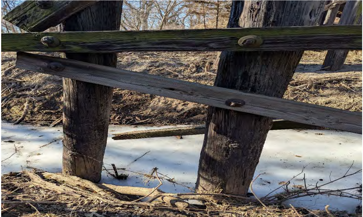
Broken X bracing and drift against piling
