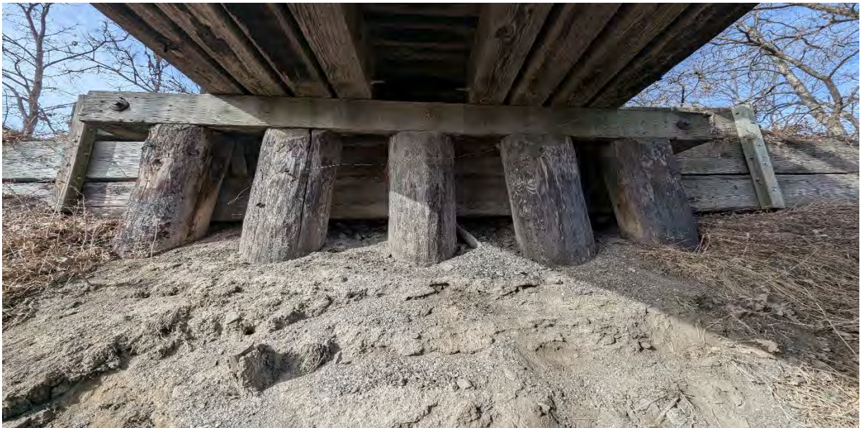
Backwall Bent 1, undermined
