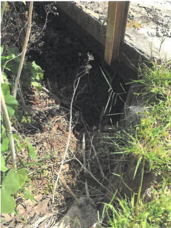
Erosion at Elm Street bridge.
