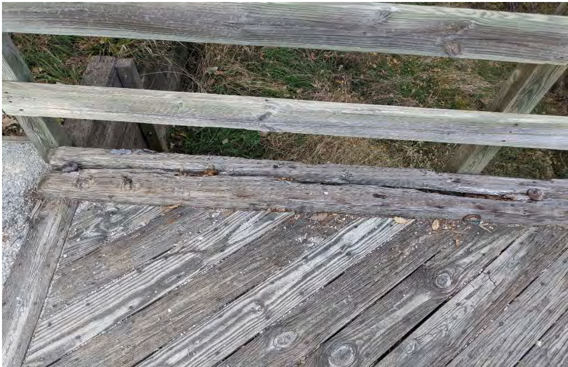
Rotten timber guard to be replaced
