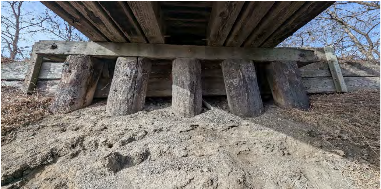
Backwall Bent 1, undermined
