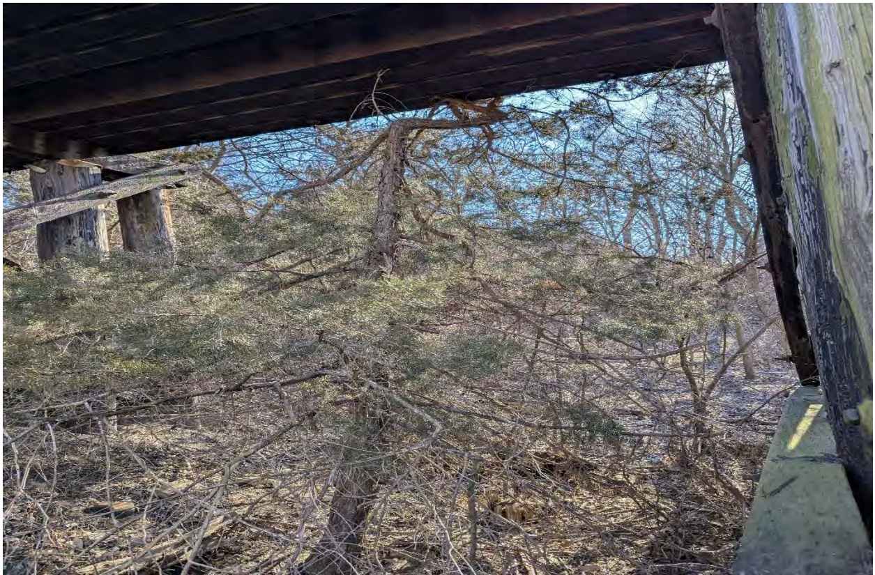
Tree growing into bottom of bridge
