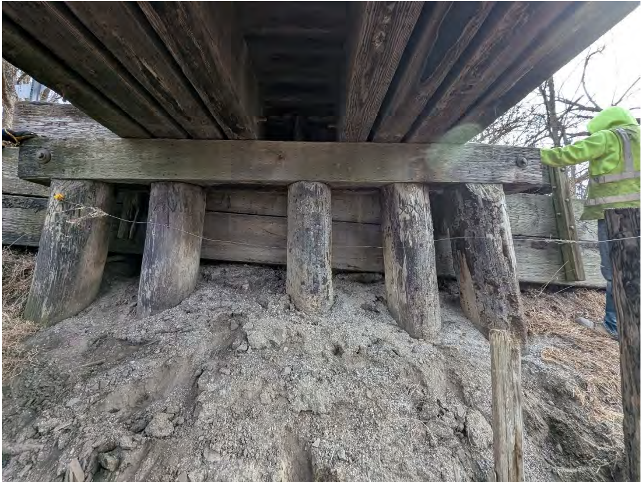
Undermined backwall bent 6
