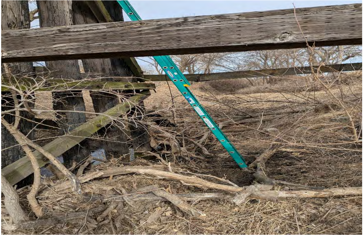
Broken Girt and drift span 4
