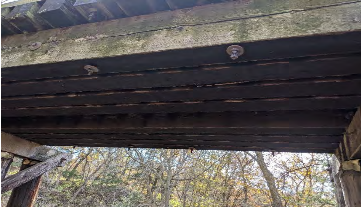
Span, longitudinal crack stringer #1
