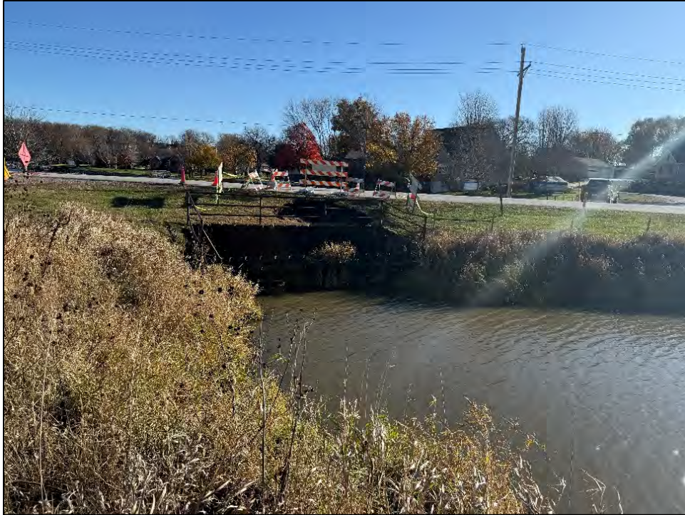
Photo 1: Upstream end of south culvert failure.
