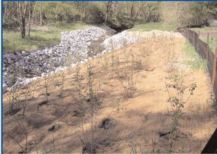
Stevens Creek stream stabilization work under way near 98th & Van Dorn streets, when completed, will look much like this earlier project.
