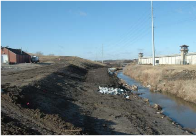
The main channel banks of Beal Slough, along the south wall of the Nebraska State Penitentiary are being widened to help reduce flooding in the area.
