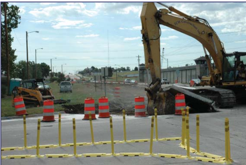
Work along Beal Slough, near the Nebraska State Penitentiary, began in September and completion is expected in the summer of 2012.
